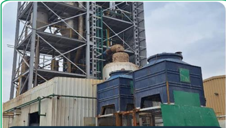
Oil processing unit
